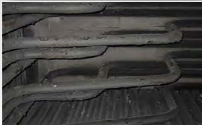
Before ceiling pipe
