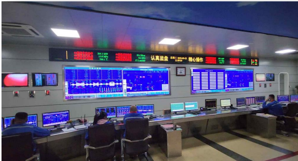
Control room of a thermal power plant
